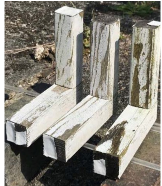
The acetylated L-joints after 20 years of exposure
